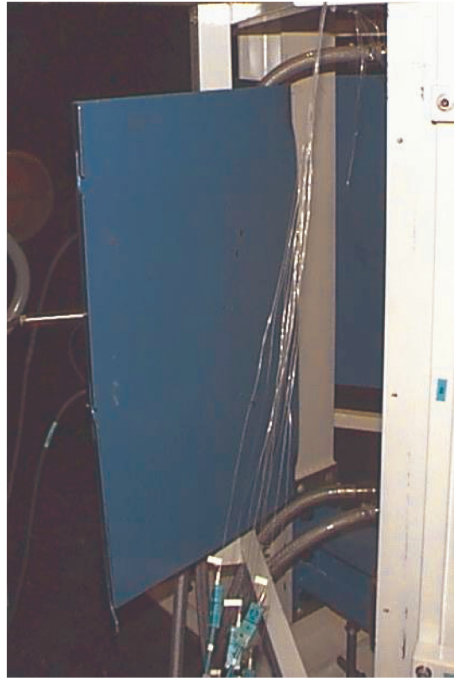
▲ Overview of the damage; view of a damaged shield
