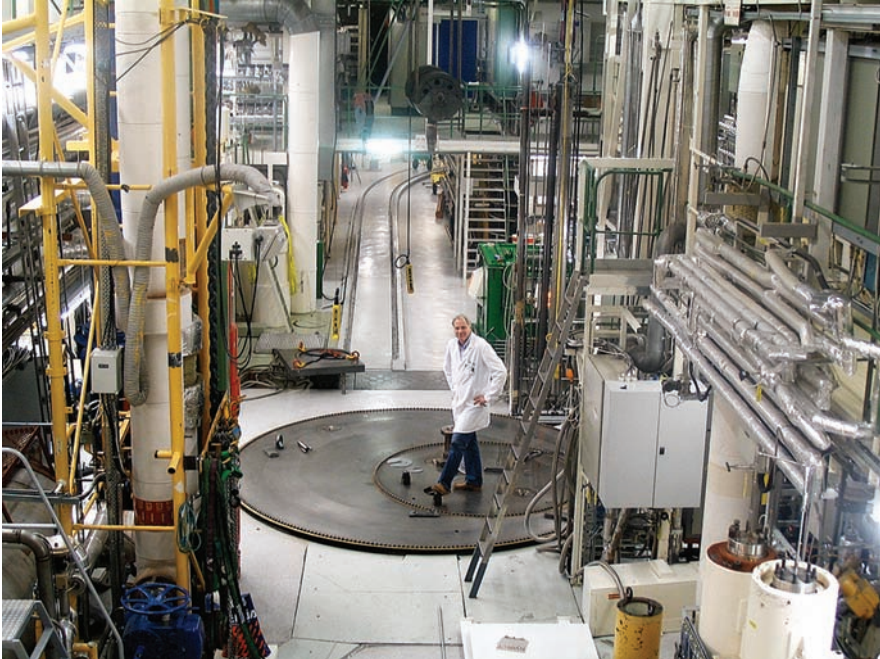
Figure 11.2 View of the Halden reactor hall. © IFE (Institutt for energiteknikk).
