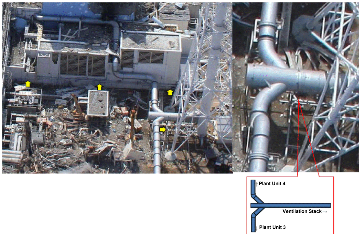
Figure 5-13 - Gas treatment system of reactors 3 and 4
